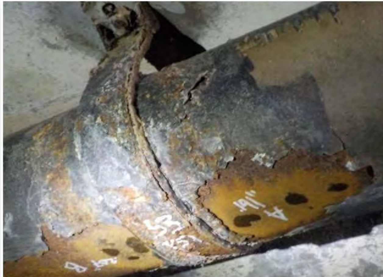
Lowest Pipe Thickness Reading .191" Spool 3
