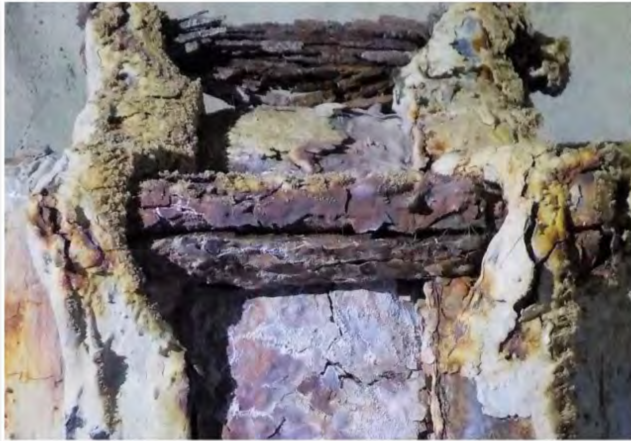
Typical Coupling Bolt Damage Spool 3 & 4
