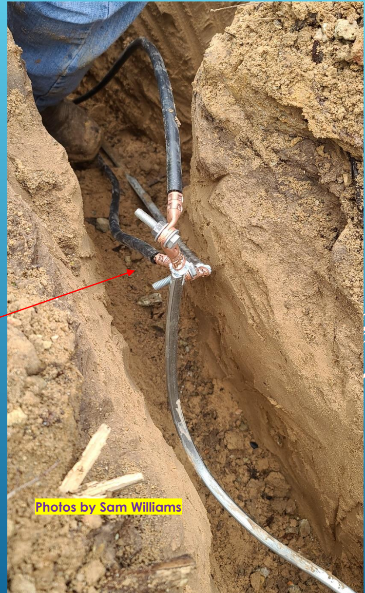
Zinc Ribbon Connected Back to De-Coupler, and to Pipeline Leads
