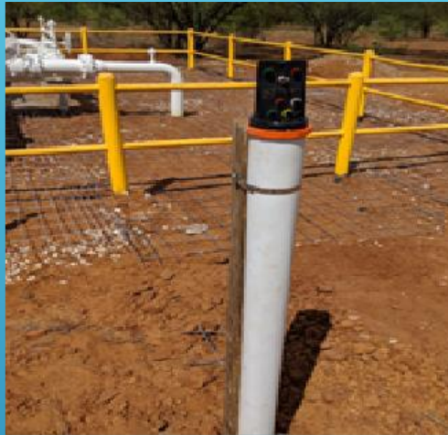
Dead-Front Test Station On Pipe Outside Pig Receiver Pen
